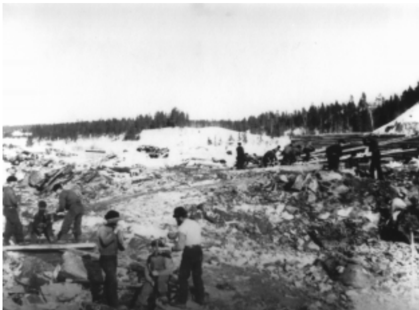
FIGURE 7. Clearing the rapids and building of a twin-faced box boom, probably at the turn of the century (1900), in Degerforsen and the eddy just above Kallholmen .
