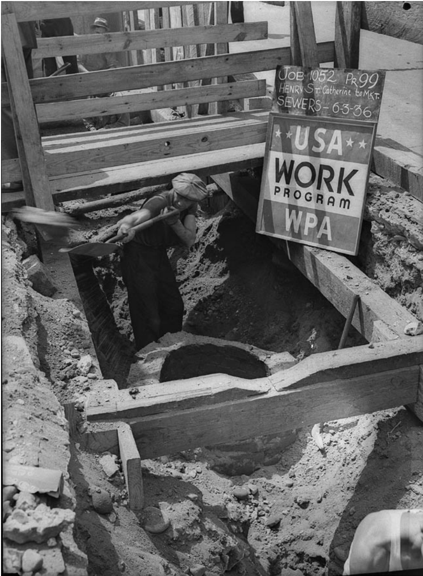
Figure 5. During the New Deal era, many WPA projects such as this in Manhattan improved sewerage and sewage treatment. Photograph courtesy of the U.S. National Archives and Records Administration (NARA).
