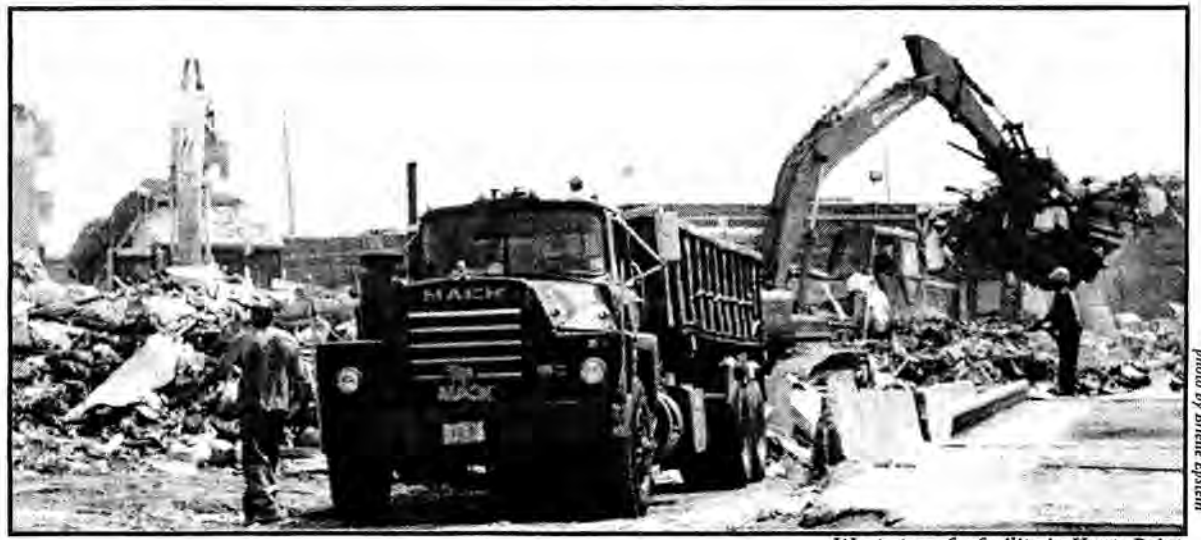
Waste-transfer facility in Hunts Point.
