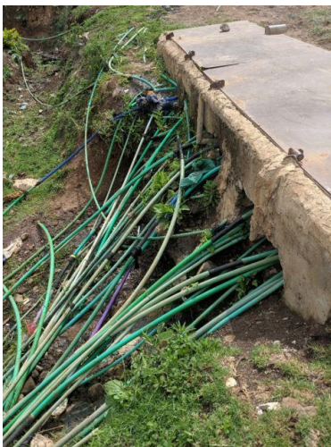
A “chamber”: a locked concrete box with legal metered connections to the grid, Kibera 2021.
