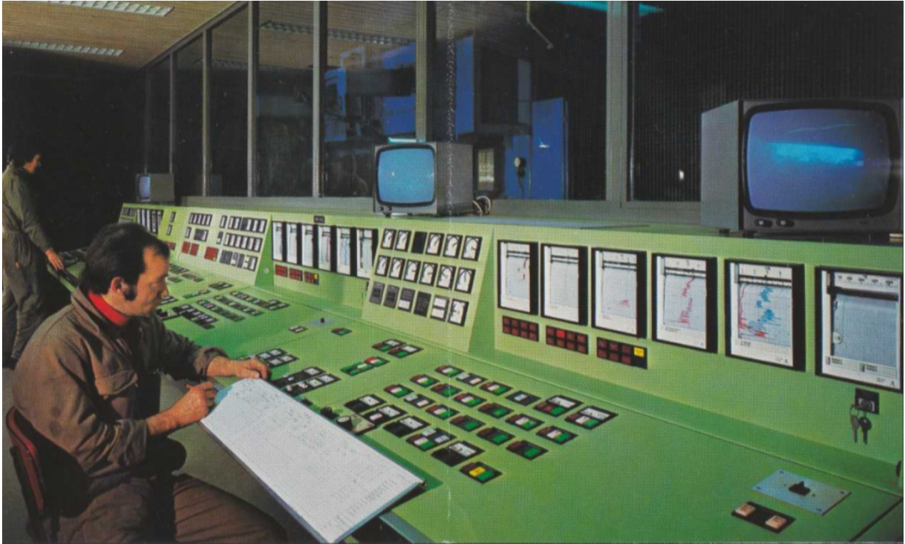
The control room from where the landscape is monitored.
