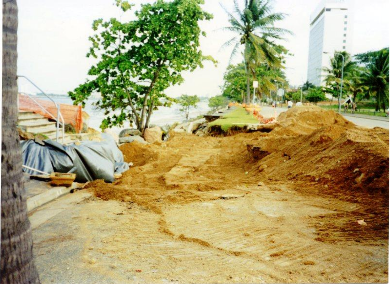
Photograph showing damage to Townsville's Strand, 15 January 1998.
