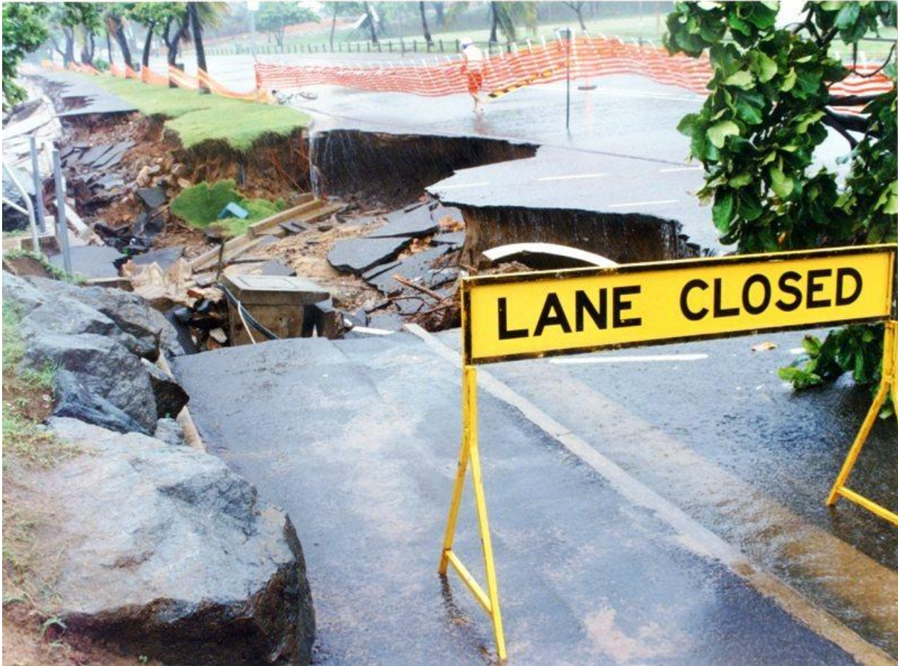
Photograph of damage to Townsville’s Strand from heavy rain, January 1998.
