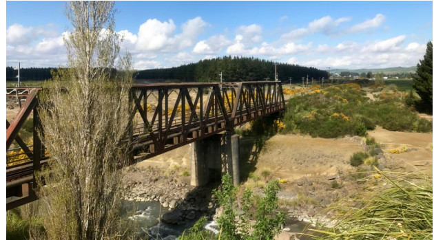
The new bridge built after the disaster still carries the North Island Main Trunk Railway across the Whangaehu River. The ill-fated express approached from the opposite bank.
