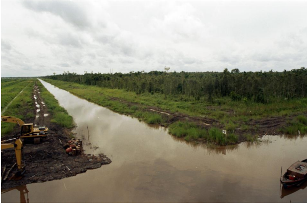
View of canals excavated in peat forest for Mega Rice Project, Central Kalimantan, 1997
